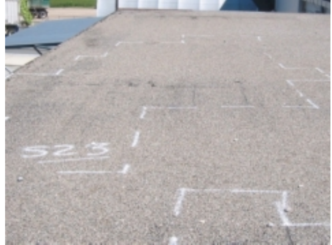
Regular photograph of roof, wet area identified.
